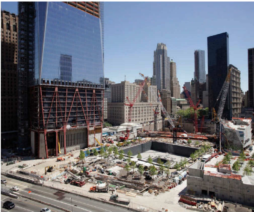
THE FREEDOM Tower rises above Ground Zero in New York City. New technology where designers work side by side with the builders can raise the risk of professional liability exposures.
